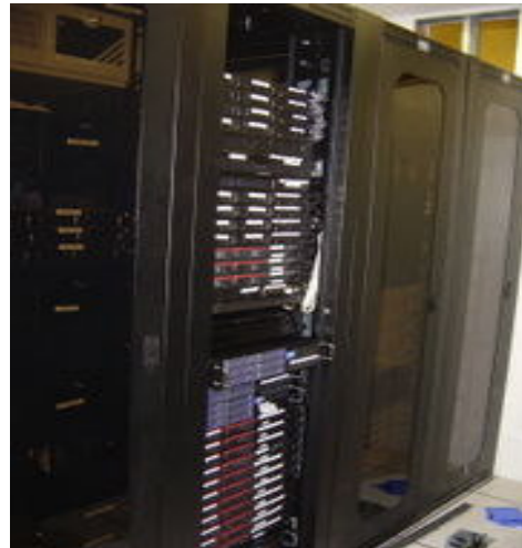
Figure 1: A row of 19-inch racks in a modern server farm.
