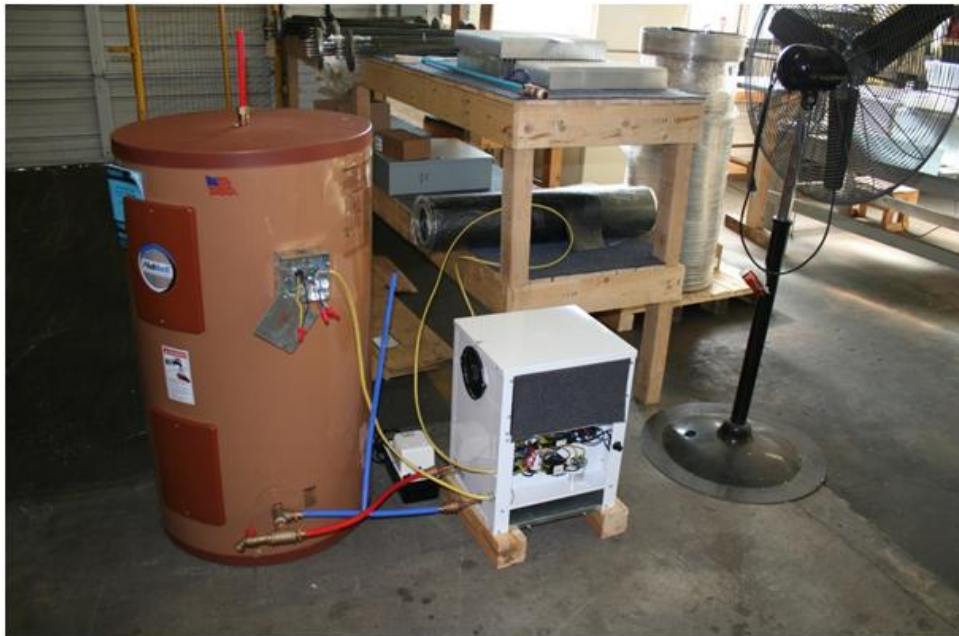
Figure 1. HPWH (R060) and Tank Prior to Installation
